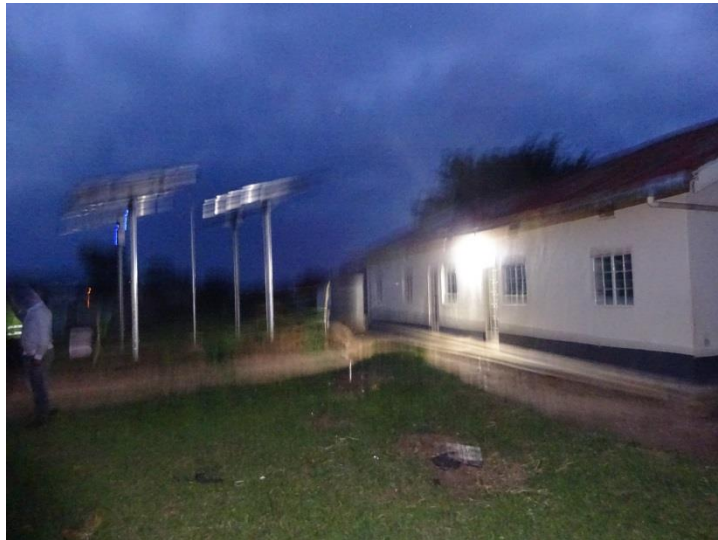
Pole mounted solar Array at one of the electrified HCs
