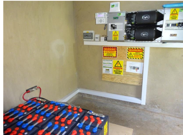
Battery bank and Inside the Solar House
